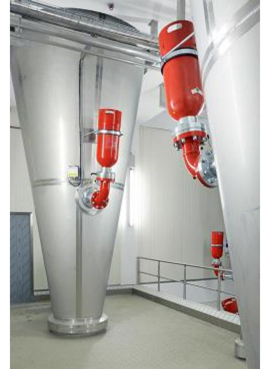
Explosion Suppression Extinguisher
